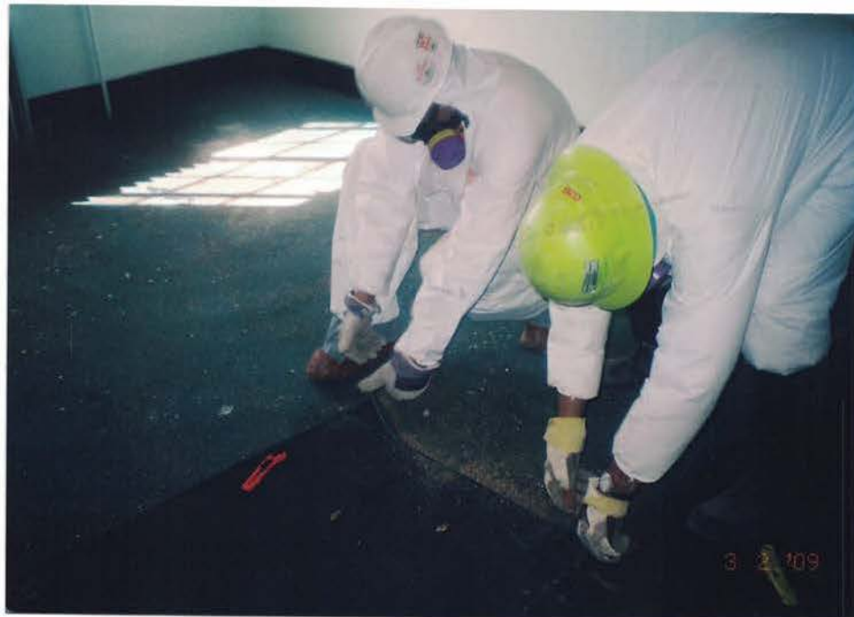
Photo #16: Carpet was cut and removed by Spray workers. Note that the personal protective equipment (PPE) donned by the Spray workers consists of high-efficiency particulate air (HEPA) filtered respirators, disposable Tyvek suits, hardhats, and gloves. The carpet was disposed of as nonhazardous solid waste. Viewing down, and to the northwest.
