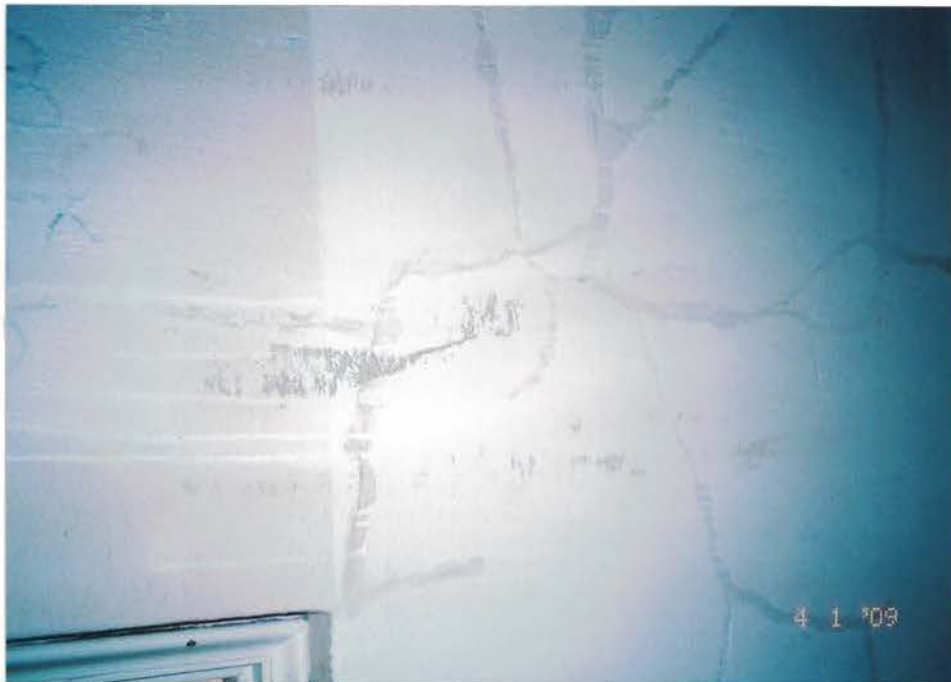
Photo #30: Loose and flaking paint was scraped, cleaned, and encapsulated in order to stabilize the LBP walls for repainting by others. Viewing southwest.
