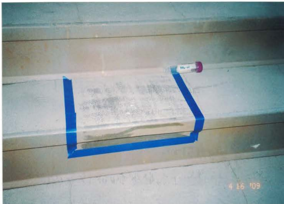
Photo #40: Post-abatement wipe sample B116-21, collected from the 2nd floor south stairwell stair tread, is reported with 170 \text{ ug}/\text{ft}^2 which warrants additional cleaning by Spray. As per the HUD regulations, the entire concrete stairway must be recleaned. Viewing down, and to the east.
