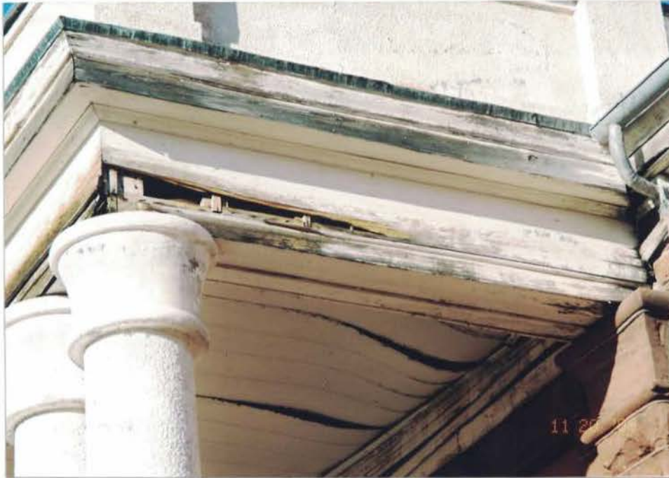
Photo #5: Water-damage on the portico roof has resulted in buckling of the wooden ceiling, and deterioration of structural components. The portico roof drains eastward toward the main roof, and is not equipped with scuppers or gutters. Viewing up, and to the northeast.
