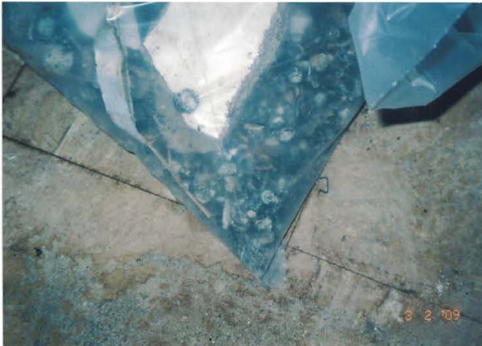
Photo #18: Bat guano, contained within a 6-mil poly waste bag, was shoveled from the floor of the attic. Note that the asbestos-containing 12" x 12" vinyl floor tile/black mastic has not yet been abated. Viewing down.
