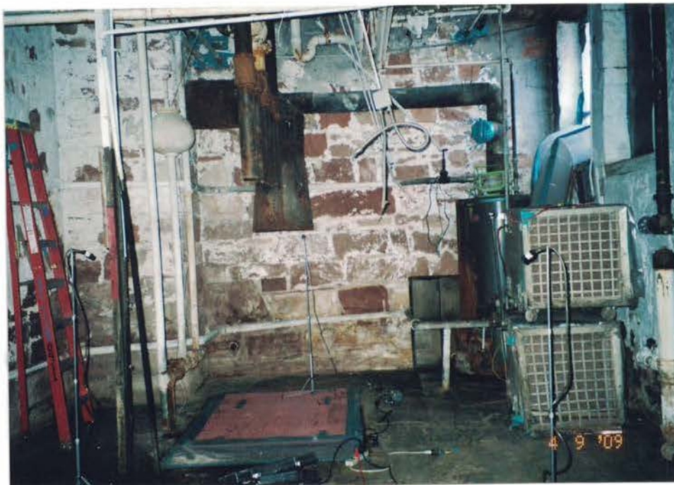
Photo #32: Post-abatement clearance air samples, collected inside the boiler room, are reported < 17 structures per square millimeter ( \text{str}/\text{mm}^2 ) of asbestos which is well below the AHERA clearance standard of < 70 \text{ str}/\text{mm}^2 . Following the stripping of TSI, the boiler was removed for recycling of the metal. Compare this to photograph #9. Viewing north.
