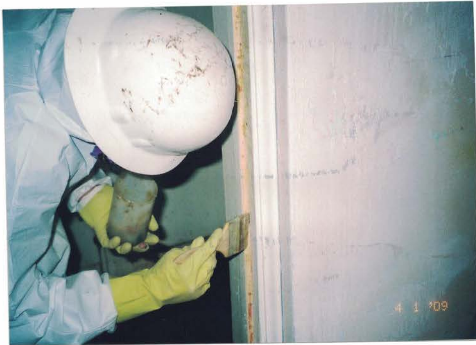
Photo #27: Spray workers apply a paint stripper to LBP on friction and impact surfaces at the location of a removed door system. Workers applied the stripper with a paint brush before manually scraping it off with a chisel. Viewing southeast.
