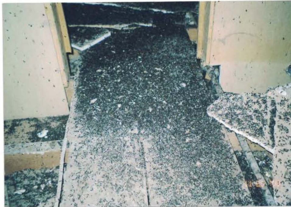
Photo #4: Copious amounts of rodent droppings cover the entire attic floor, and are up to 6-inches deep in some locations. Drywall debris, construction debris, and fiberglass insulation inside the attic have to be bagged and removed prior to biocleaning. Viewing down, and to the north.
