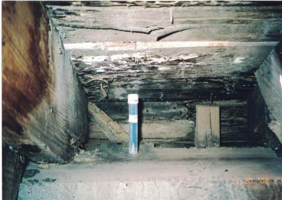
Photo #6: Inside the attic at the location of the portico roof, there is water-damage, structural damage, staining, and mold contamination. Swab sample 08TEC304-01 is reported with elevated counts of fungal mold that warrants removal of contaminated materials. Viewing west.
