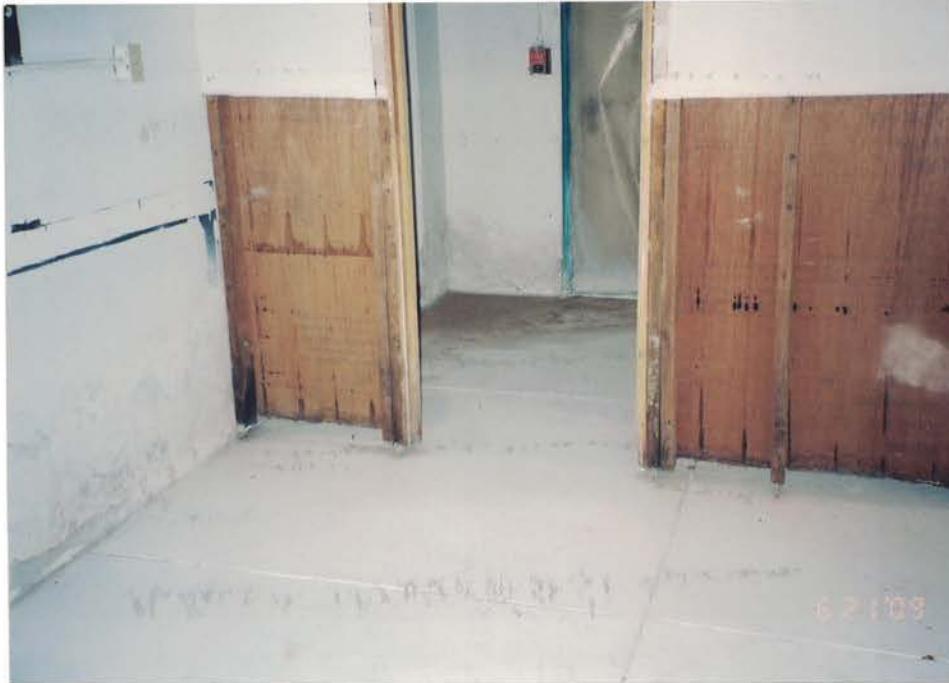
Photo #63: Mold contamination present inside the northwest room inside the north basement recreation room, has been removed. Note that the opened and biocleaned wall cavities have been cut to a height of 4 feet. Viewing southeast.
