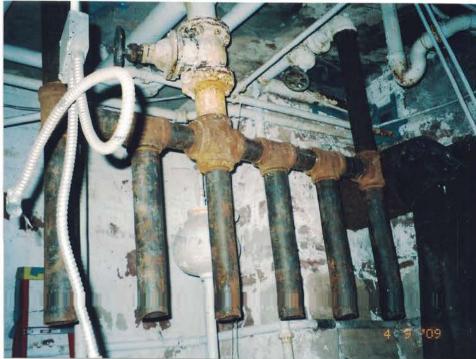
Photo #35: TSI from the boiler pipes was removed and the area cleaned prior to the cutting of the metal pipes, and removal of the boiler. Note the thoroughness of the removal. Viewing up, and to the northwest.
