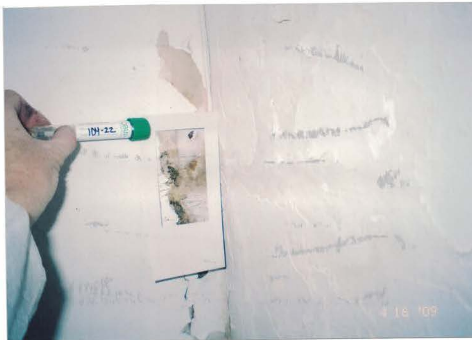
Photo #48: Swab sample 09TEC104-22, collected from visible mold on the south recreation room southwest wall, is reported with a total spore count of 21,000 c/cm 2 which warrants additional work by Spray at this location. Viewing southwest.
