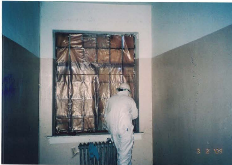
Photo #15: Spray workers constructed critical barriers consisting of 6-mil polyethylene (poly) plastic around windows, doors, and HVAC registers to maintain a negative air pressure differential inside the building during the abatement activities. Viewing north.
